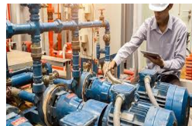
Fig 5. Pump station safety.
